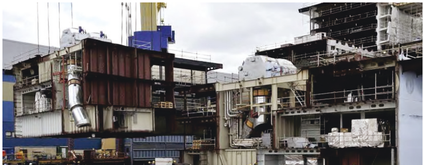
Figure 5. An outfitted block is being lifted to the hull during the hull assembly period.
