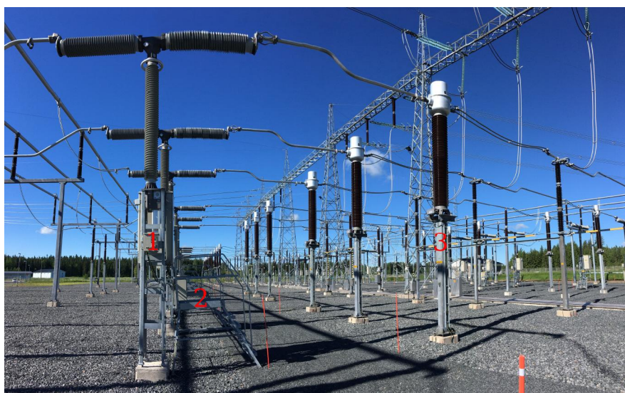
Figure 1: Overview of the studied area. Objects of interest numbered: 1. Circuit breaker 2. Service platform 3. Current transformer.
