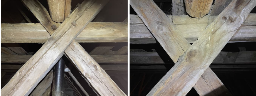
FIGURE 11 Different types of joints between scissor beams and the Collar Beam B. On the left it can be seen that there is an incidental drill mark which coincides with the dowel, but the dowel is intact PHOTO BY LAURA LAINE (2024)
