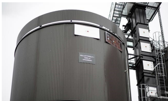
Figure 34: 1000 m 3 pellet silo in Salmisaari power plant, Helsinki (Helen 2016)
