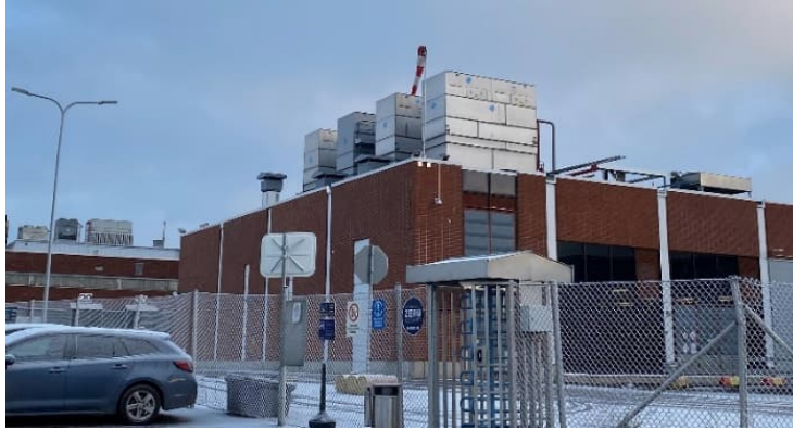
Figure 25: Ammonia cooling compressor exhaust heat condensers on top of the technical center (number 7 in figure 21)
