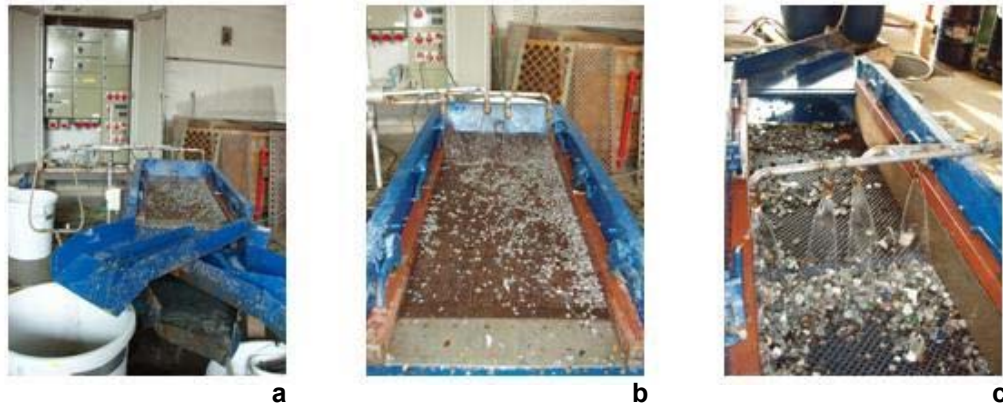
Figure 6-4 Wedag MN 917/1 screen a) overview b) process c) washing
