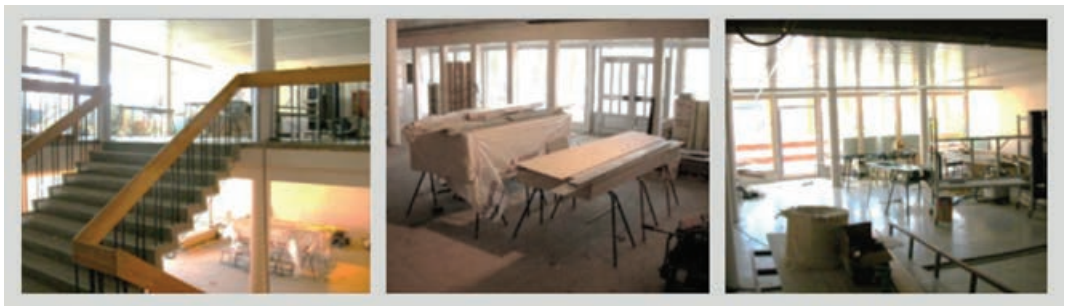
Figure 3.1 : A (left), B (middle), C (right): Entrance area in the secondary school in the building process: A: Stairs. B: Ground floor. C: 1st floor.
