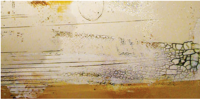
Figure 2.2: Cracked surfaces attracted attention.
