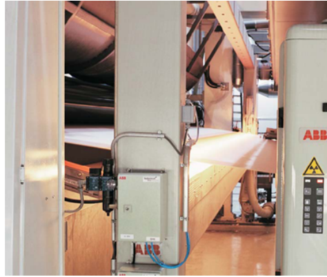
Figure 3.1: A paper web inspection machine in operation. Image courtesy of ABB Oy.
