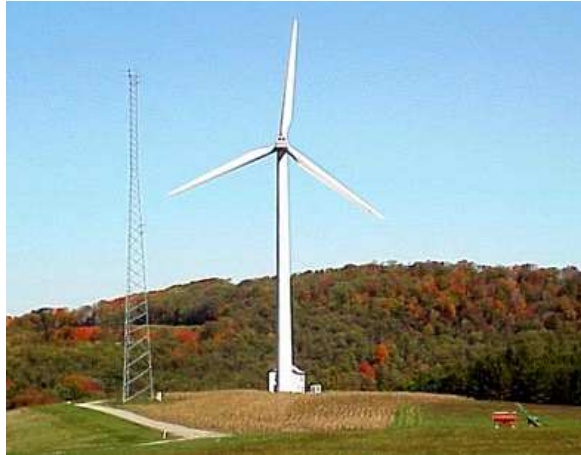
Figure 9: Wind Power turbine deployed at BS
