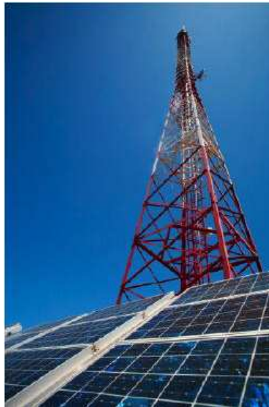
Figure 8: Solar panels deployed at BS
