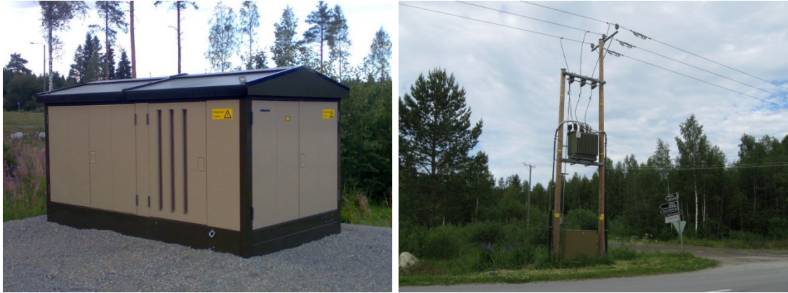
Figure 1. Pad mounted (left) and pole mounted (right) distribution substation. (Finnkumu 2019, Järvinen 2010)
