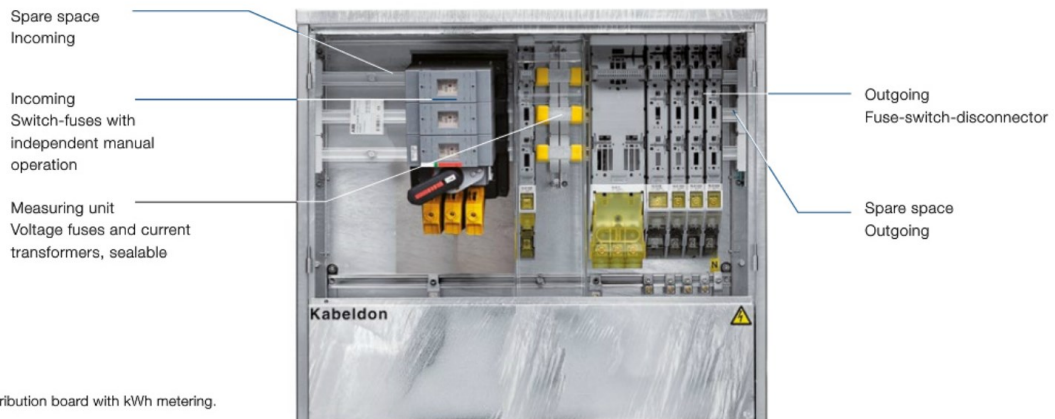
Figure 2. Contents of a cable distribution cabinet. The fuses are part of the fuse-switch-disconnectors. (ABB 2015)
