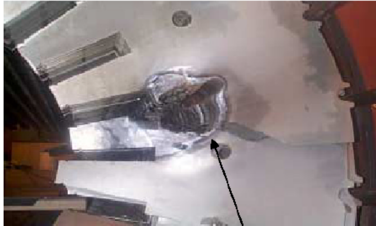
Figure 2: Inter-laminar insulation failure of stator core [13]
