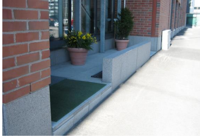
Fig.12. Step is too high.
