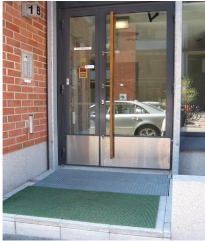
Fig. 11. Door opens in wrong direction.
