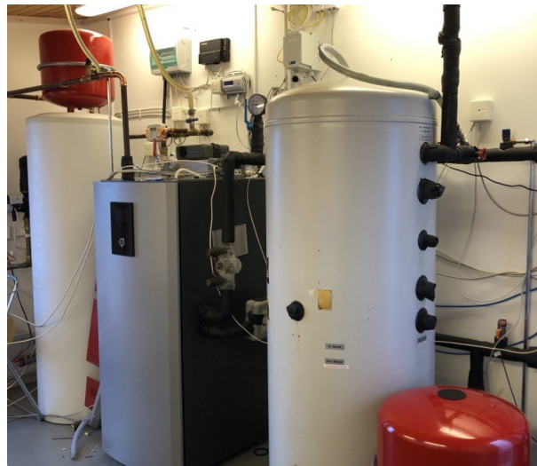
Figure 5: Heat pump used in the experiments with the cold and hot storage tanks.
