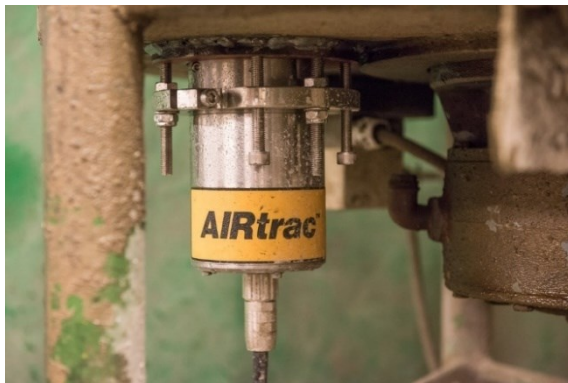
Picture 8. The CiDRA AIRtrac sensor probe installed to the mixer floor.
