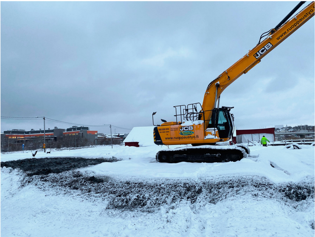
Figure 2. Site of soil circulation in Porvoo, removal of liquid clay from Porvoonjoki.
