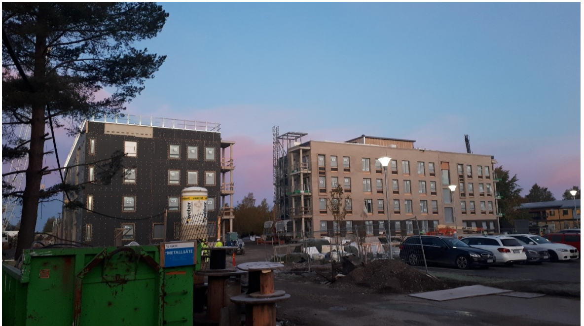
Figure 12: Picture from the site with buildings A (on the right) and B (on the left) visible
